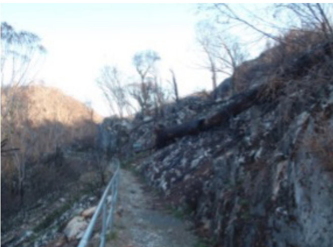
Walking track to South Glory Cave after the fire. Extensive spalling and many new fossils are now evident. The 100-year-old pines which had been blown over in a storm about 6 years previously were partially burnt in the fire and are lying above the path.
